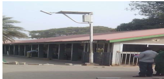
Plate 4: Solar Powered Street Light
